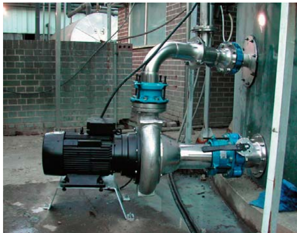
Dry-installed AirJet in tannery effluent aeration tank
