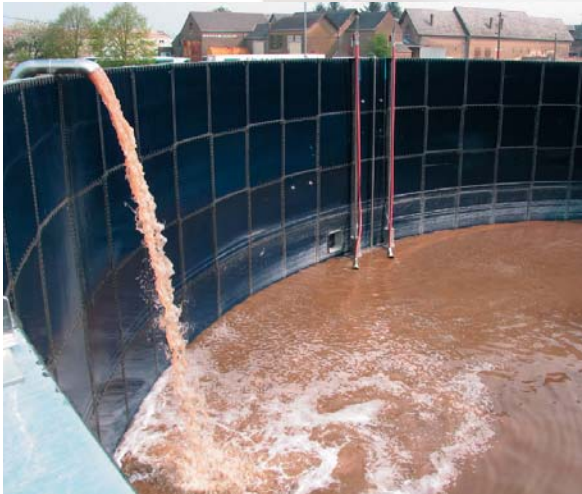
Submersible AirJet for odor alleviation in abattoir wastewater
