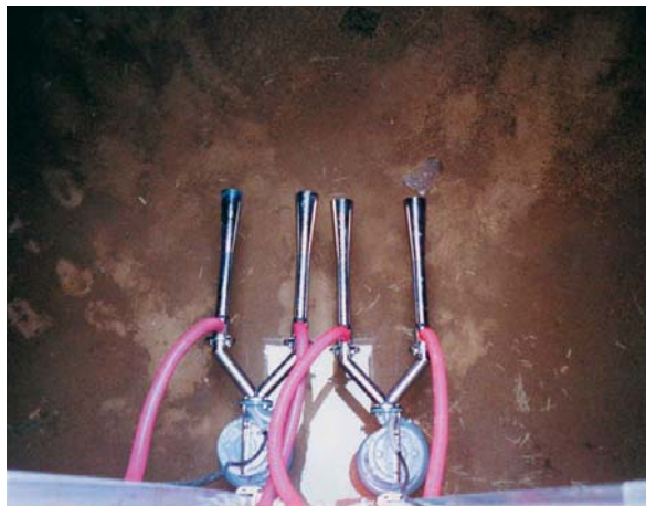
Submersible AirJets in leachate tank
