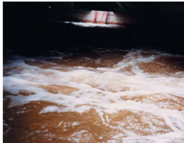
Submersible AirJets in leachate tank
