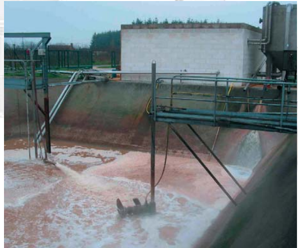
Combined system of submersible AirJet and submersible mixer in equalization tanks from vegetable processing industry
