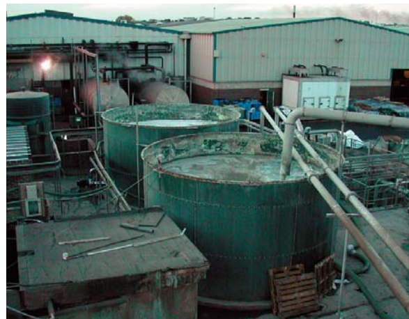
Dry-installed AirJet in tannery effluent aeration tank
